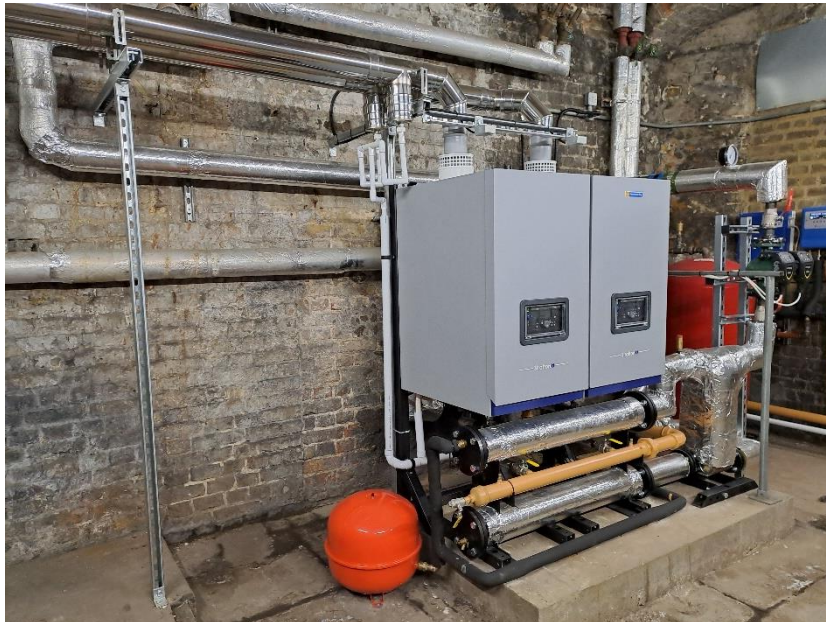
St Dunstan in the West: two new energy efficient condensing boilers were installed in the church's crypt.
