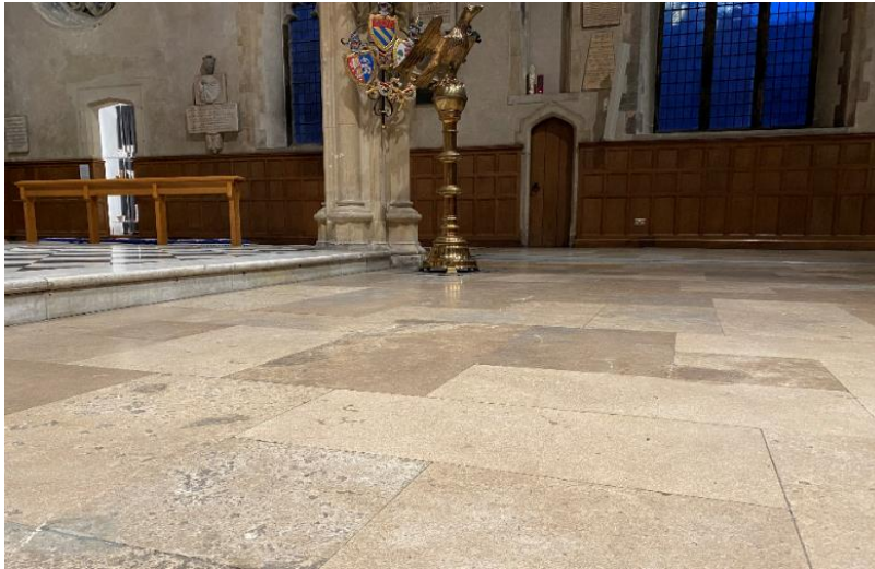
St Giles' Cripplegate: repairs to the main nave floor have now made it safe and level
