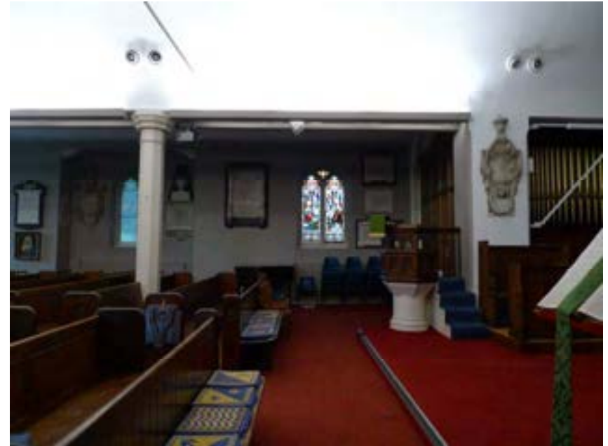
View of the location of the proposed new door opening (east window of the north aisle)
